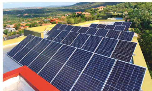
Solar Electric Panel
